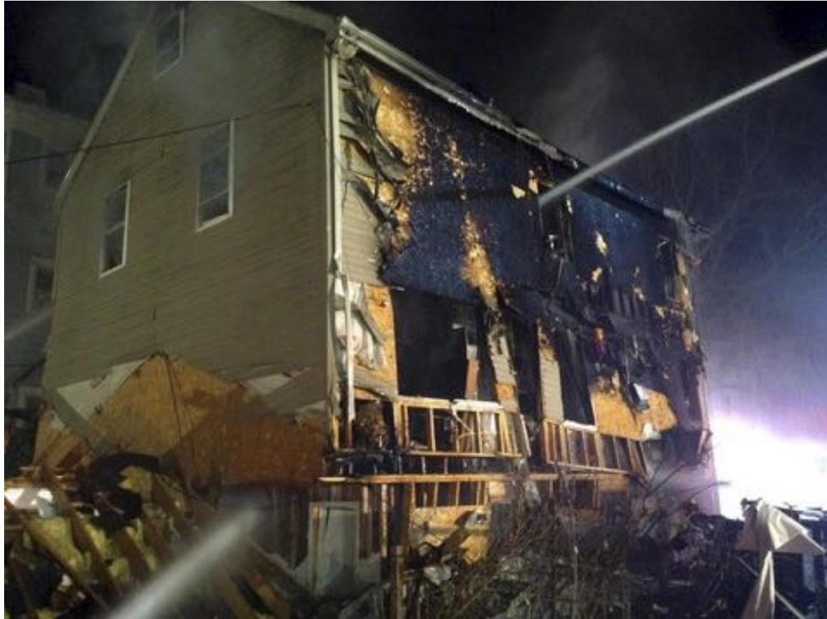
April 2014: 12 hurt in Dorchester gas leak explosion
